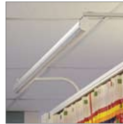
Overhead Aisle Lighting
